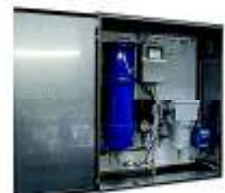
60 lit/min system in an enclosure
